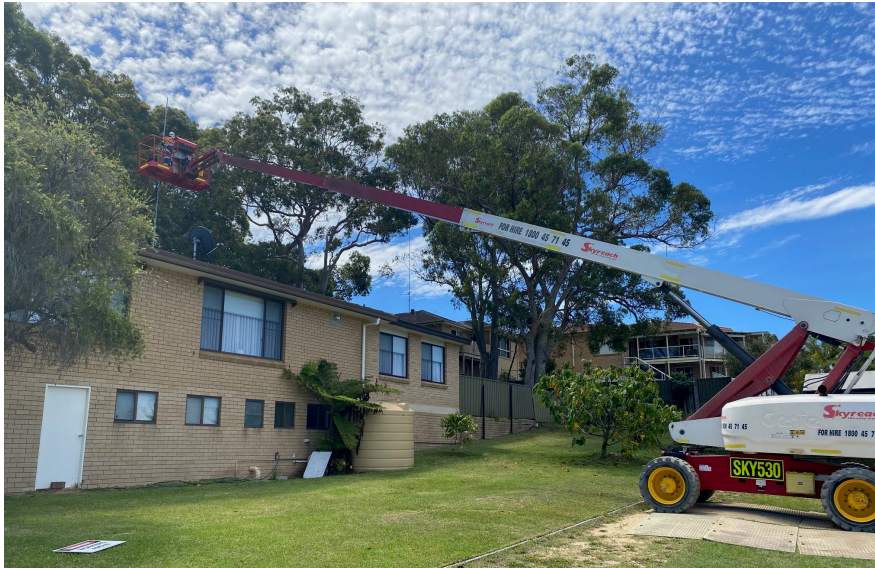
Photos of the work done to replace the antenna on the manse:
